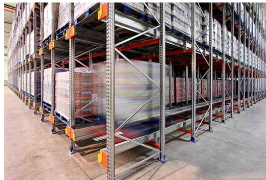
Figure 5. Ar shuttle system for compact semi-automatic storage.
