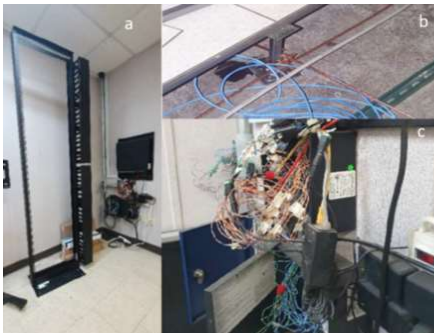
Figure 1. a) Rack with its organizers, b) Physical ground installation, c) Wires marked before disconnecting
