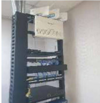
Figure 5. Order of devices in the rack
