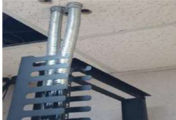
Figure 2. The wiring distributed by the envelopes until reaching to the distribution.
